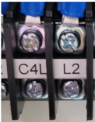
Pump POWER wire
