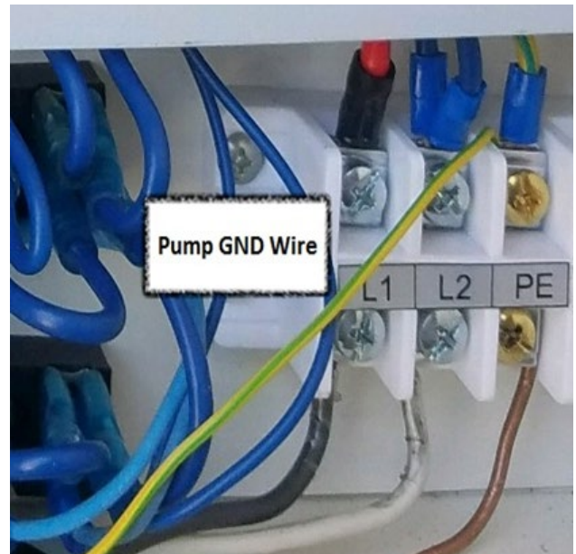
Pump GROUND wire.
