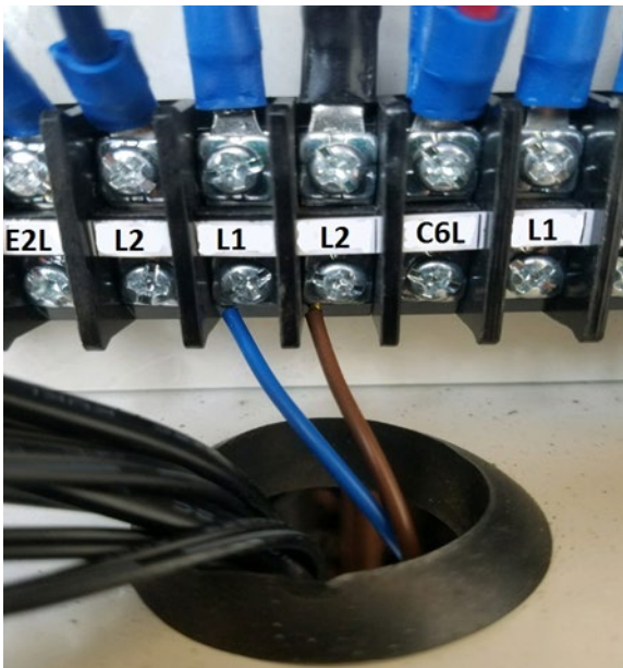
Pump POWER wires.
