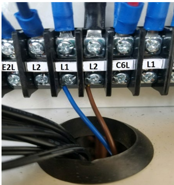
Pump POWER wires.
