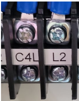
Pump POWER wire
