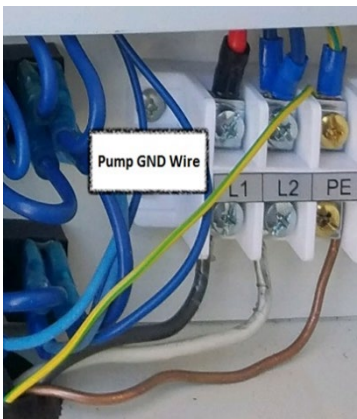
Pump GROUND wire.
