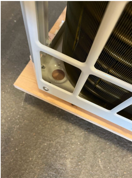
Figure 1: Shows location of drain hole without hose adapter
