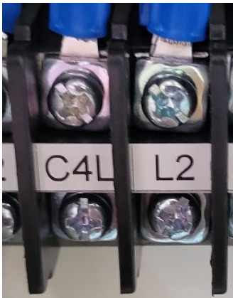
Pump POWER wires
